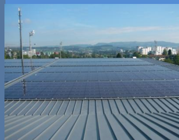
204.4 kWp Bossard Arena, Zug
